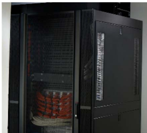
Installed on AR3340 enclosure
